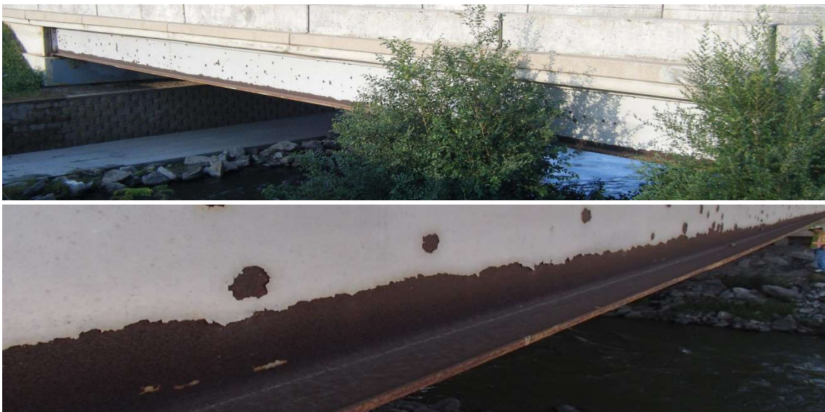
Figure 4.2 Bottom flange deterioration along the girder
