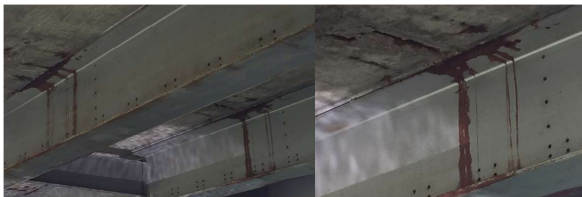
Figure 4.4 Entire girder section deteriorated below the cracked slab
