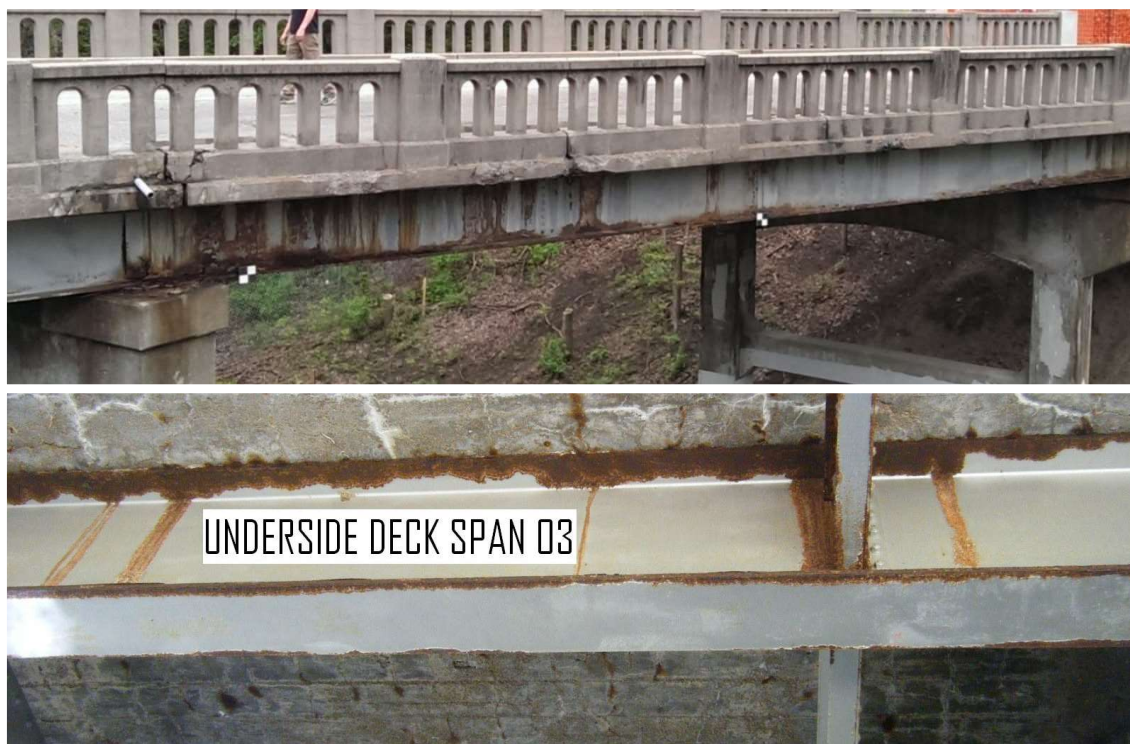
Figure 4.3 Deterioration pattern where entire section of girder is deteriorated
